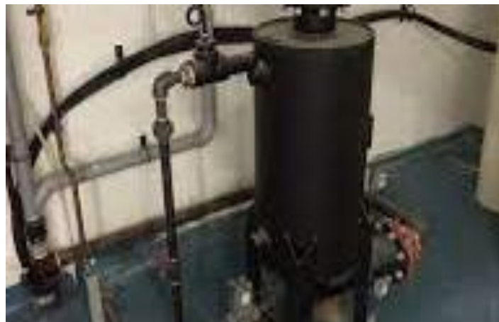
Blowdown Heat exchanger
