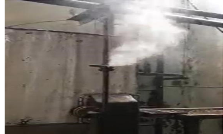
Steam Leak at the valve
