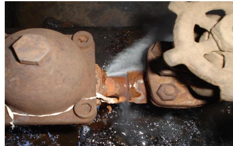
Steam leak at the steam trap
