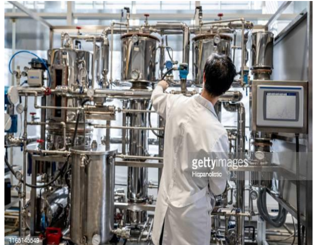
Pneumatic systems installed in a Pharmaceutical plant
